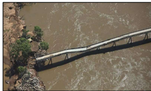
Figure 6: Damaged Bridge into Fitzroy Crossing 2
