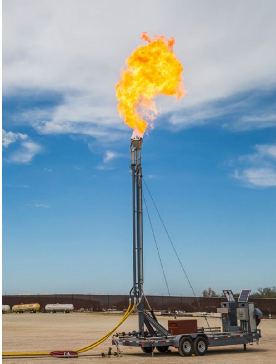
Figure 4-3: Multi-Stack Vertical Flare for low-pressure and high-pressure gas
