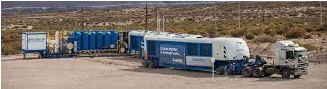
Figure 4-5: Well head gas capture via Mini-LNG (Source: CryoBox)
