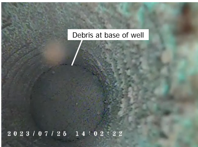
AB1S debris build up on casing wall and bottom of well.
