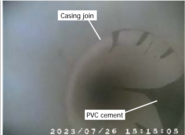
VNB4S casing joint showing PVC cement.
