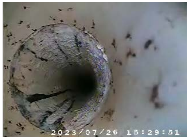
VNB4D insect debris at dry casing joint 6.7 m btoc.
