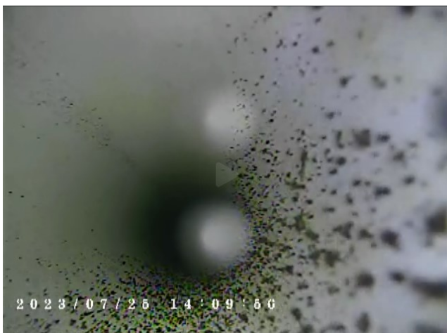
AB1D insect debris build up on casing wall below SWL.
